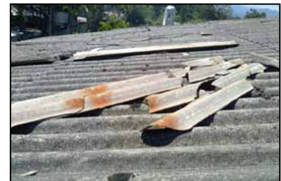
Roof tiles blown off by tornado November 1, 2013
